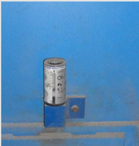
Drip lubrication on chain
