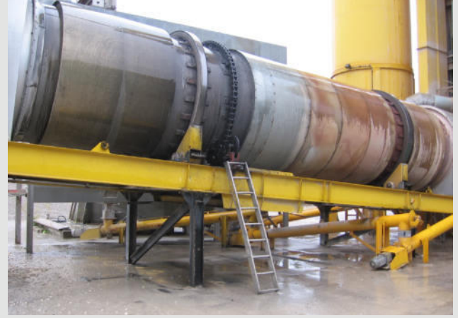
Drum dryer - chain drive
