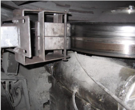
Pressure roll cement factory
